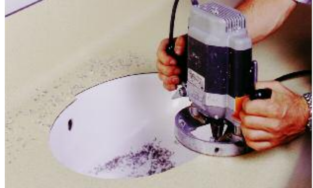
4. Mill the projection of the Compact Laminates flush on the visible side with a manual surface miller (angled miller!).
